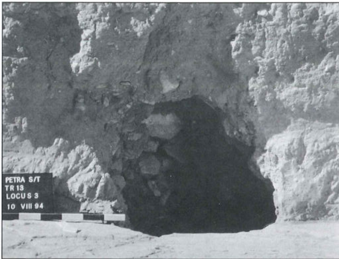
6. Petra Southern Temple, Trench 13 collapse, 1994, facing south.
