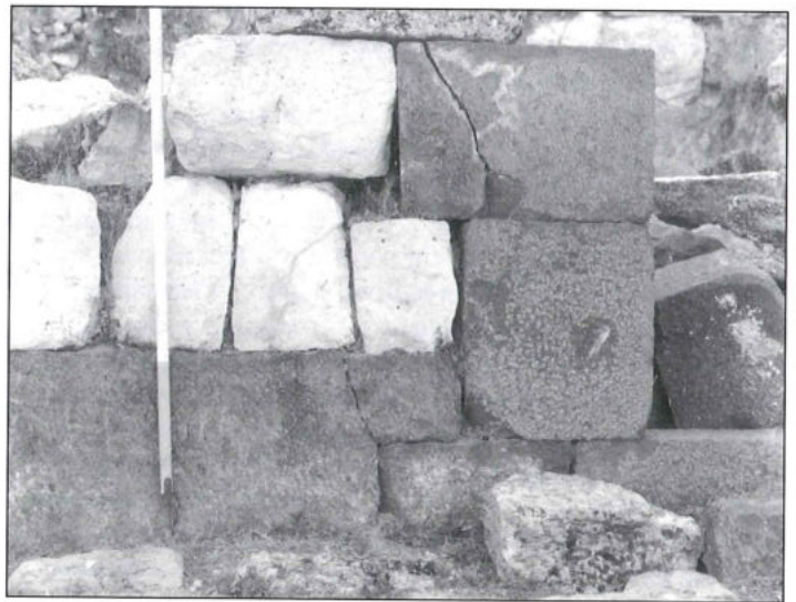
2. Construction Type IB. Façade of one of the rooms east of the atrium.
