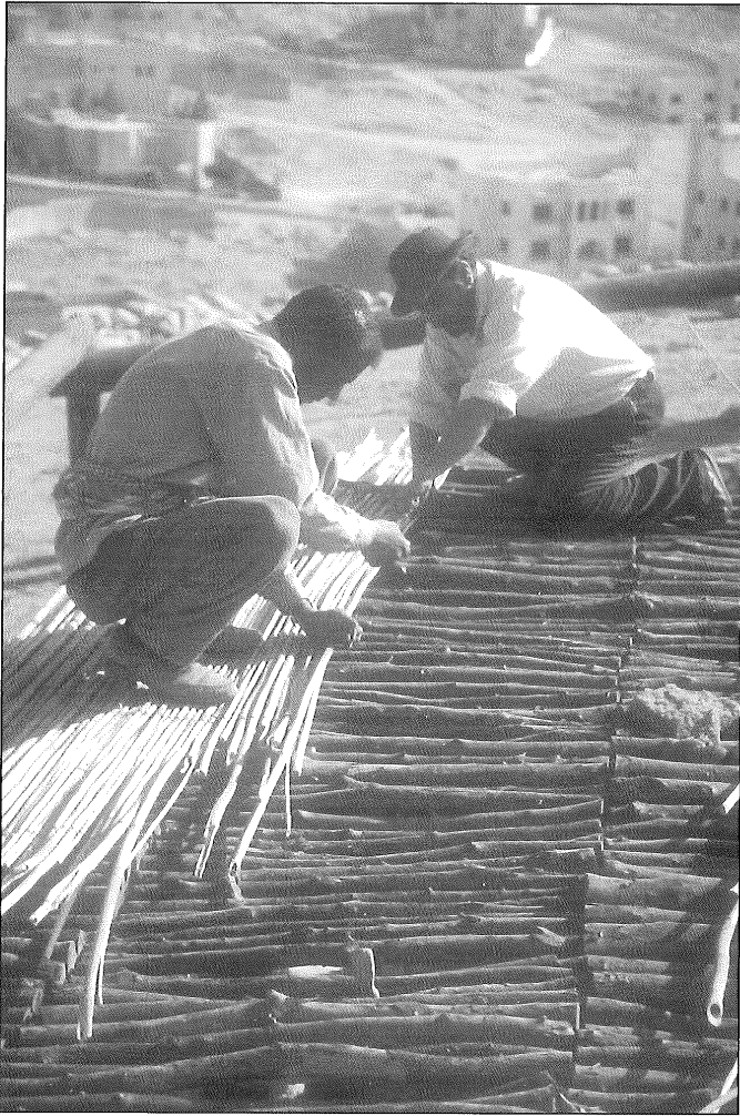
7. Reeds transported from the Jordan Valley being installed on the partially reconstructed al-'Umayri house.
