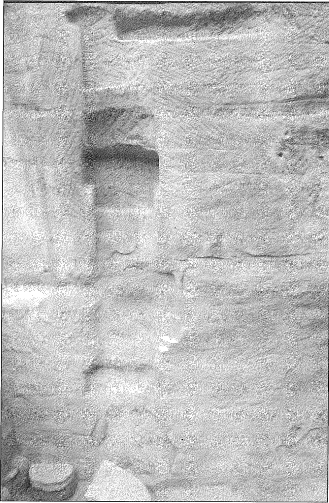
3. Wādī Farasa East, lower terrace. SW corner of northern portico of Soldier Tomb's complex with rock cuttings for first column and roofing (S.G. Schmid).
