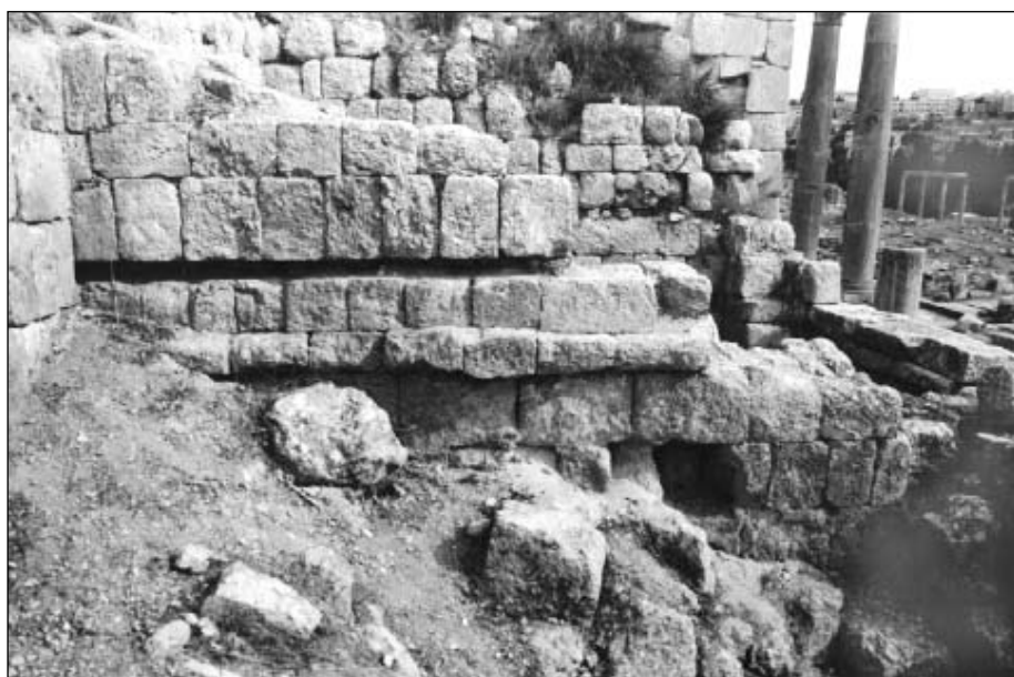
4. Interior of room G, showing corbeling for upper floor and put-log hole for the second phase upper floor ( ca. 0.50m below earlier floor) (WB).
