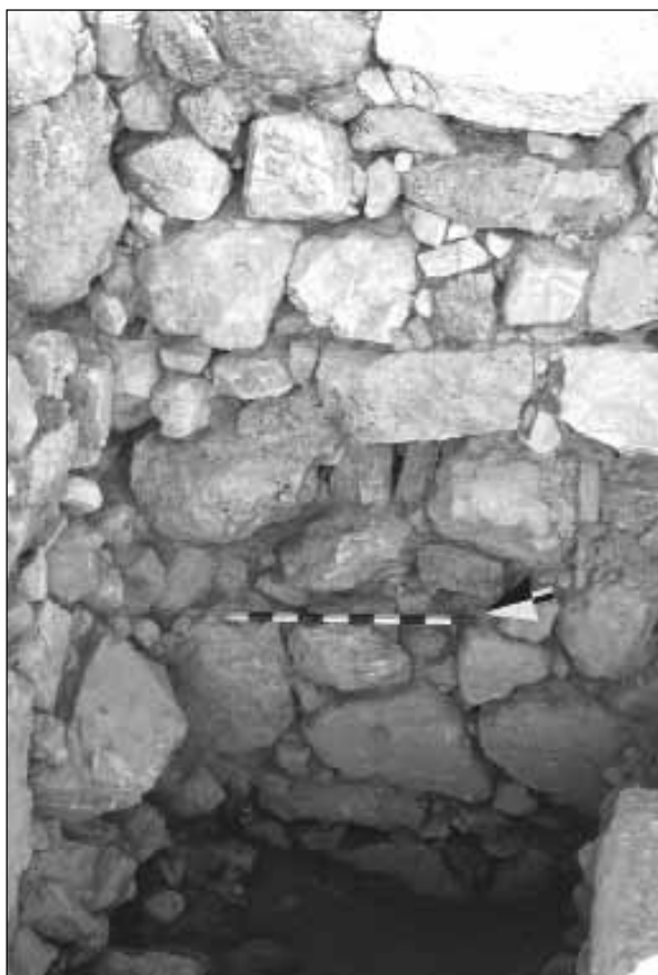
6. Tall al-'Umayri: Field A, Stratum 12: A small portion of the stone perimeter wall that protected the south-western portion of the site; at left is the later Iron 1 wall also visible in Figure 5.
