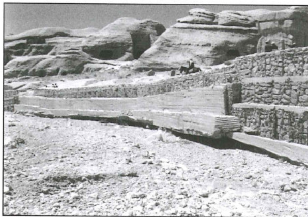
28. Erosion cavity below the foundations of the sidewalls of Wādi Mūsā, in the Bab as-Siq area.
