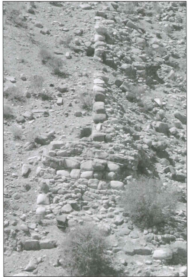
15. The dam below Mughur an-Naṣāra, view from the wadi bed towards the north. At the bottom, the full thickness of the dam, exceeding 6m, is visible. The narrow stone line above is part of the water channel which crossed Wādī al-Maṭāḥa on top of the dam.
