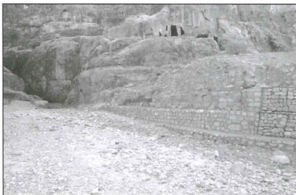
14. The retention wall reinforcing the southern bank of Wādī al-Maṭāḥa at the outlet of Sadd al Ma'jan. The original masonry is visible on top of the restored foundation.
