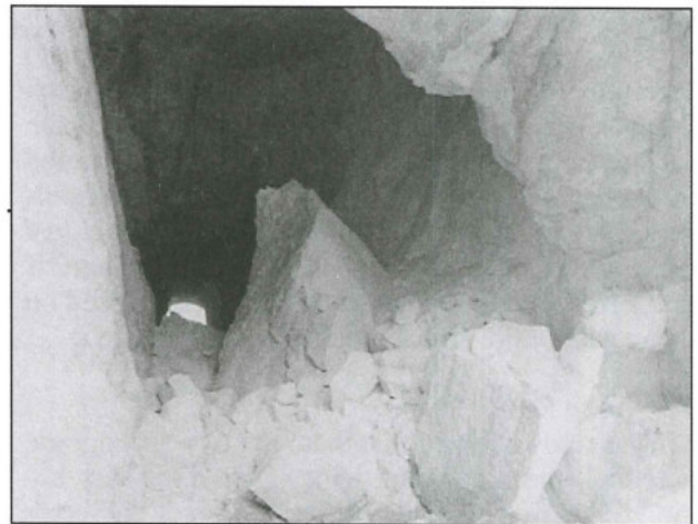
24. Tunnel entrance before clearance of rock fall.
