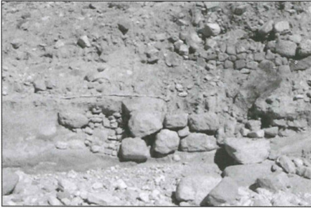
20. The northern abutment of the lowest dam in Wādī al-Maṭāḥa, which prevented runoff water from damaging the northern Nymphaeum. These fragments are now no longer visible, as they have been hidden behind a protecting wall built by the DoA in the summer of 2002.
