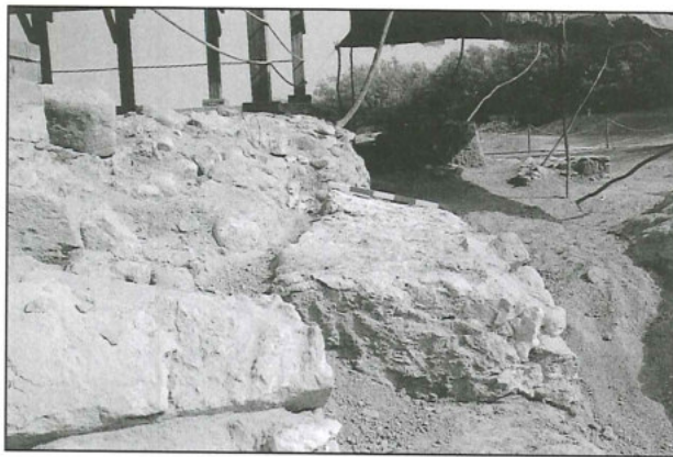
4. The bedding of the central aisle settled about 30 centimeters (from the south).
