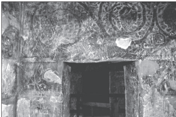
33. Vandalism in the alcove room.
