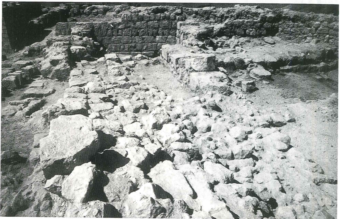
2. The US 40 and US 10 walls leaning against the perimeter wall of the tower.
