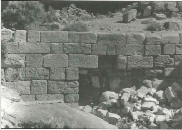
19. Petra, Wādī al-Farasa East. Main retaining wall of the lower terrace (photo by the author)
