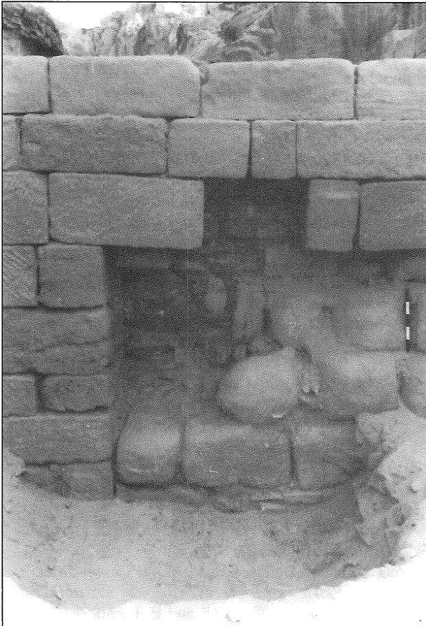
38. Lower terrace, detail of the main retaining wall from NW before restoration (Schmid).
