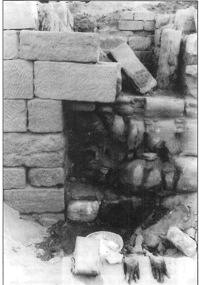
39. Lower terrace, detail of the main retaining wall from NW during restoration (Schmid).
