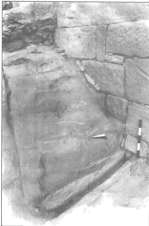
15. Lower terrace, details of construction and first cut-off water channel in front of the main retaining wall from NW (Schmid).
