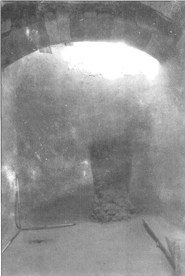
11. Cistern under room 27: view to the east of the rock-hewn communicating tunnel to the cistern under the adjacent room 22 (photo: D. Keller).
