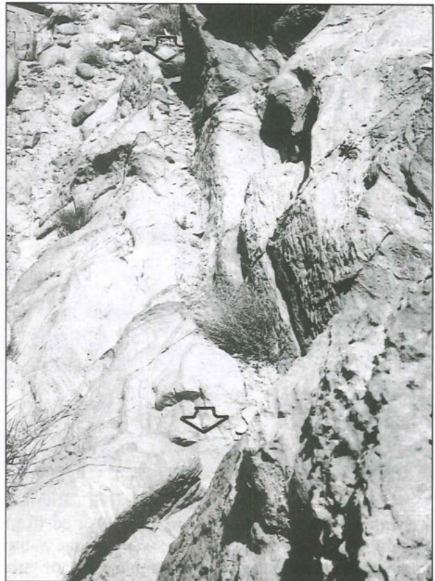
16. Section of the Šabrā conduit originally bridged by masonry or a conduit block (arrow) (1982).
