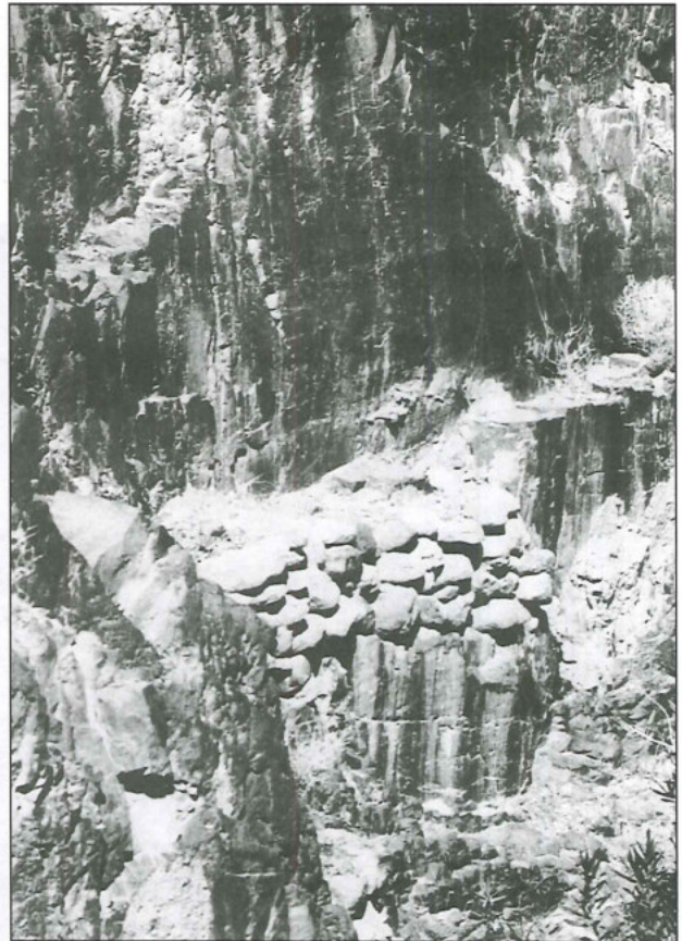
10. Remnants of a hydraulic installation in a tribu-tary rock wadi of as-Sādah. Substruction of a conduit or abutment of a dam (1988).
