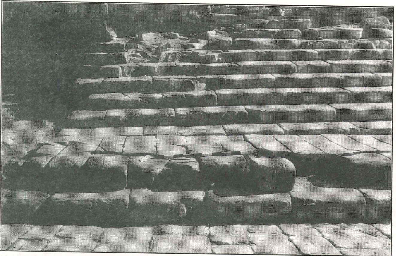
10. Propylaea Stairway leading from Colonnaded Street to Lower Temenos; lower courses, before consolidation, facing south (P. Ward).
