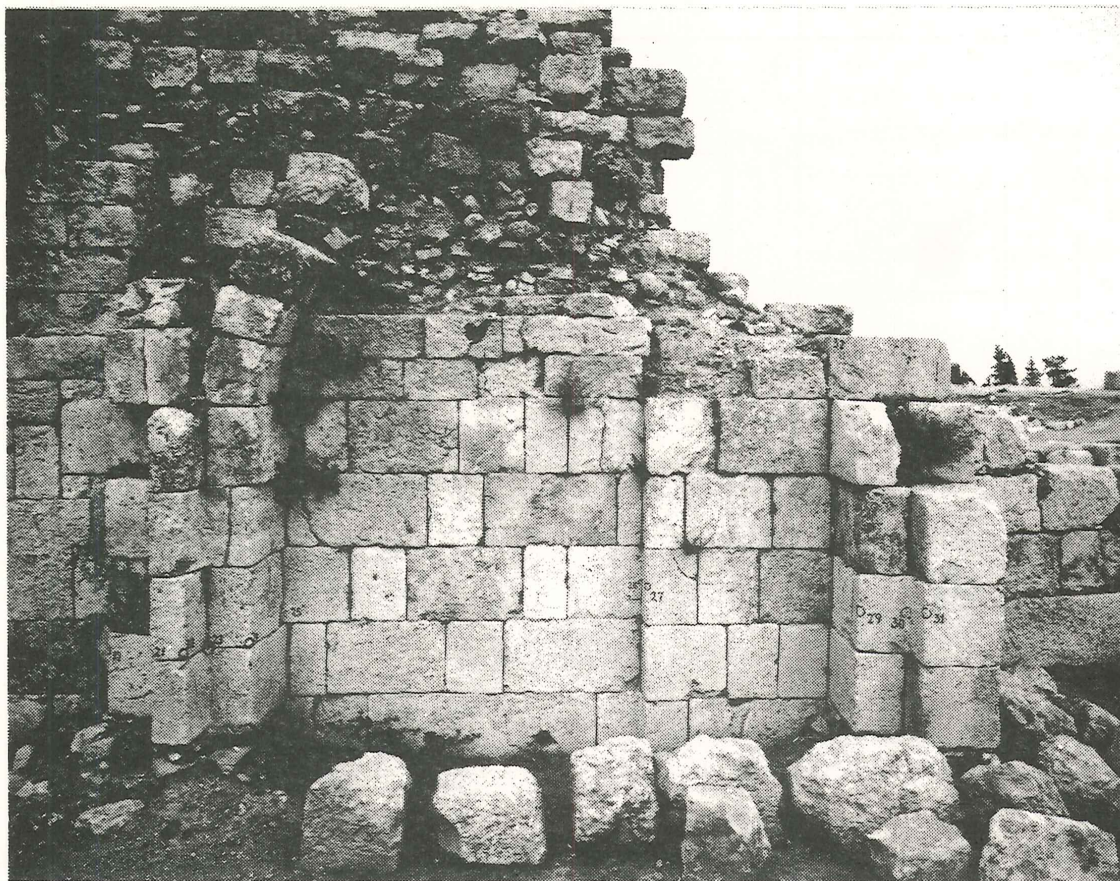
4. Detail of the foundation of the door jambs in the west wall.
