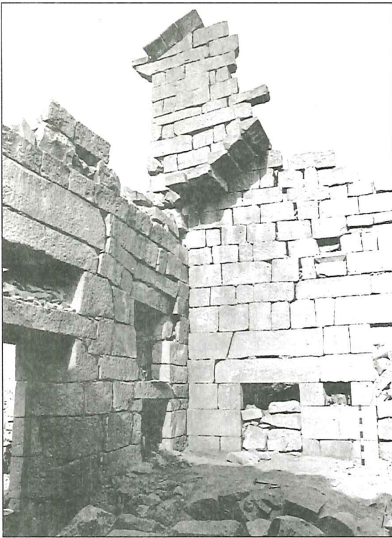
1. SW corner inside Praetorium atrium before installation of wood shoring. Note the separation of the masonry on the west wall (on the right) and the buckling of the double lintel over the window on the left (Photo by B. de Vries).
