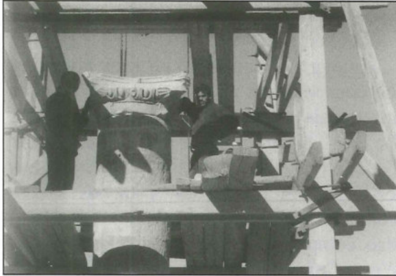
29. Lower Temenos Restoration of the East Colonnade with the placement of the Elephant-headed capital on top of the column (Dakhilallah Qublan).
