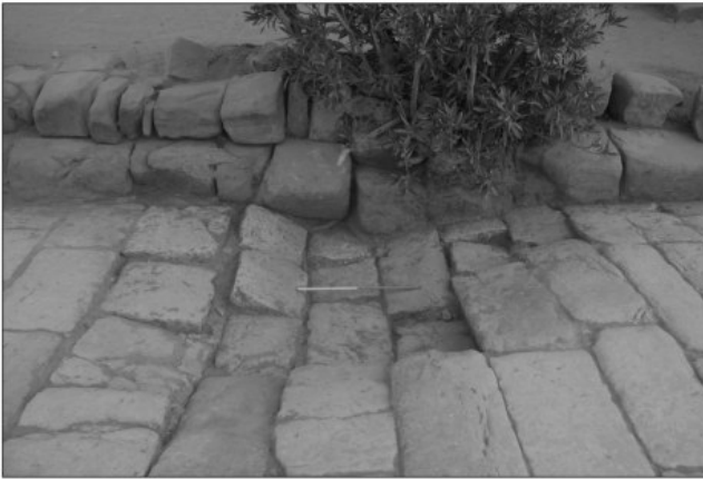
10. Collapsed southern portion of decumanus maximus towards its western end (looking south): scale=60 cm. Photo by S.E. Sidebotham.
