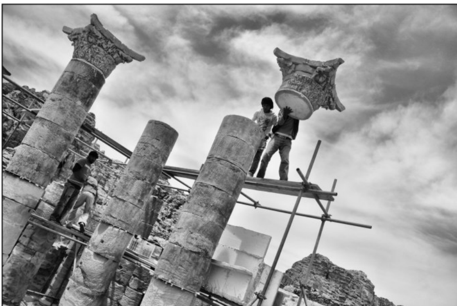
5. TWLCRM team members place the ‘faux restoration’ columns in order to test the project’s final presentation strategy. (Photo Q. Tweissi).
