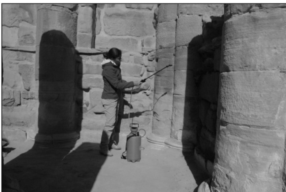
4. A member of the TWLCRM conservation team treats the north wall of the temple's cella with a consolidant solution.
