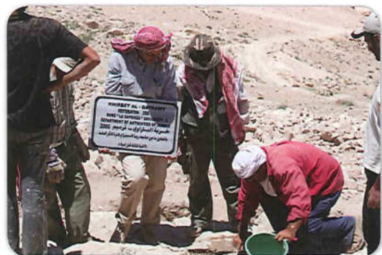
fig 5 : Restoration works undertaken during the 2006 season rehabilitating the stretch of the city-wall excavated in 2005
