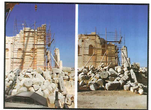
Fig. 4: Restoration of the South-Eastern Corner of the Cella: Before and After Dismantling (Photo S. Desoutter © IFPO 2008).
