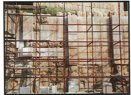
Fig1: Restoration of the North-Western corner of the Temenos Wall (Photo J. Brunet © IFPO 2009).
