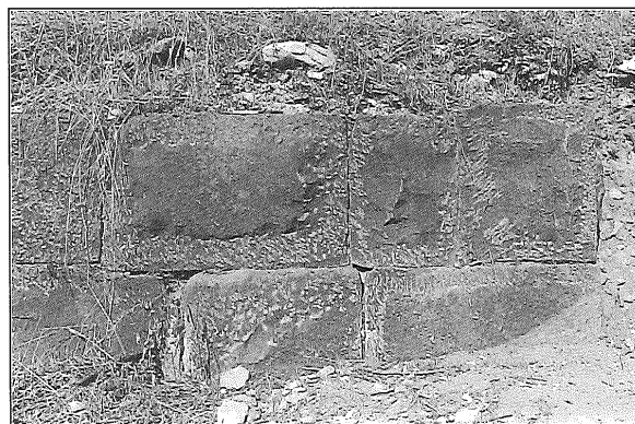
10. South corner of the façade of the vaulted rooms with rusticated stone blocks.
