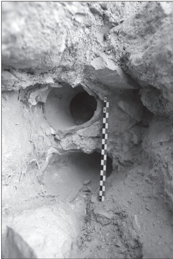
15. Water pipes in the southern wall of the warm room/ wasṭānī (©Mission Dusaq 2015/R. Elter).
