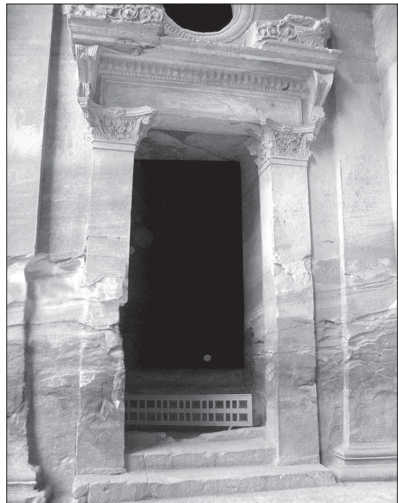
3. View at the doorway in the southern wall of the entrance hall of al-Khaznah, showing the heavy erosion of the sandstone, reaching almost half of its height. This erosion is due to the crystallization of salts during the evaporation of the rising ground humidity in the void of the stone structure in the warm seasons (Photo U. Bellwald).
