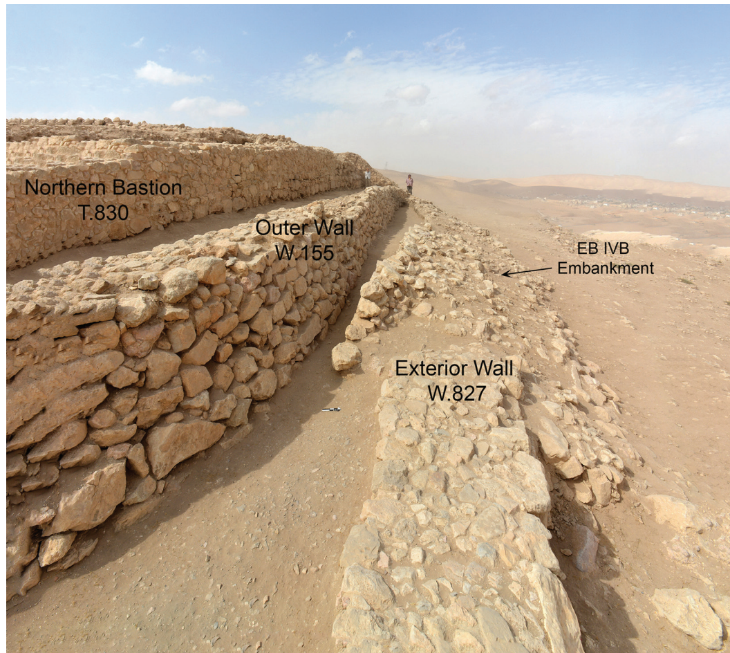
8. View of Exterior Wall W.827 and Outer Wall W.155 with its outer battering face and the two corridors, L.858 (between Bastion T.830 and Outer Wall) and L.862 (between Outer Wall and Exterior Wall), seen from the south-east.
