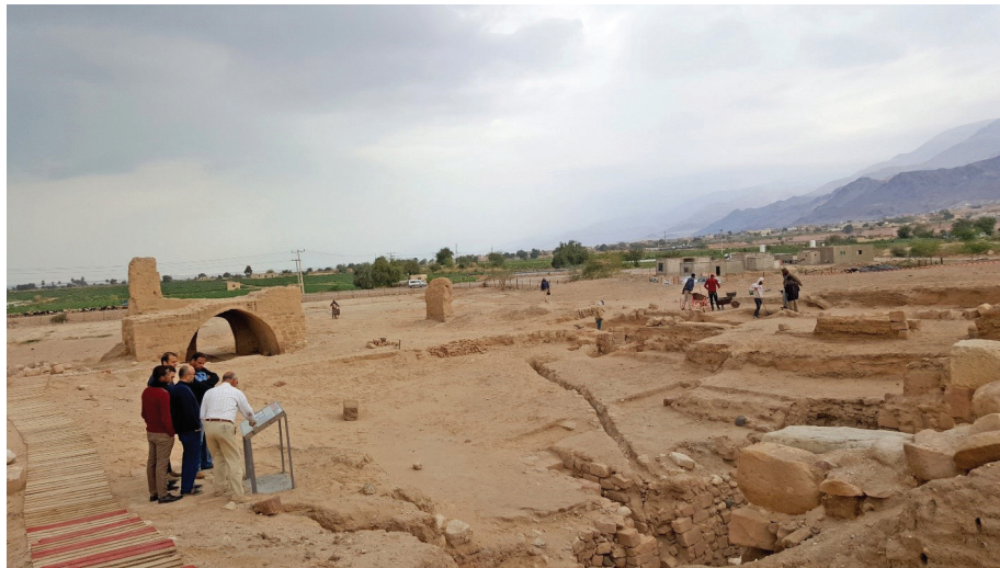
4. Local community members work on site development in Ghawr aş-Şāfi. Photo by Barbara A. Porter.
