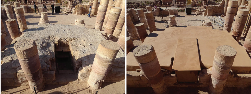
20. Before and after the application of a protective mortar capping on the Cella podium in 2017. Photos by Franco Sciorilli.
