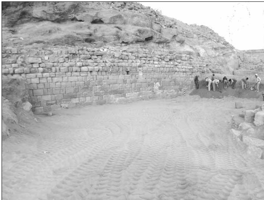
2. Excavating the sandy fill overburden between the island-pavilion (lower right) and south wall.
