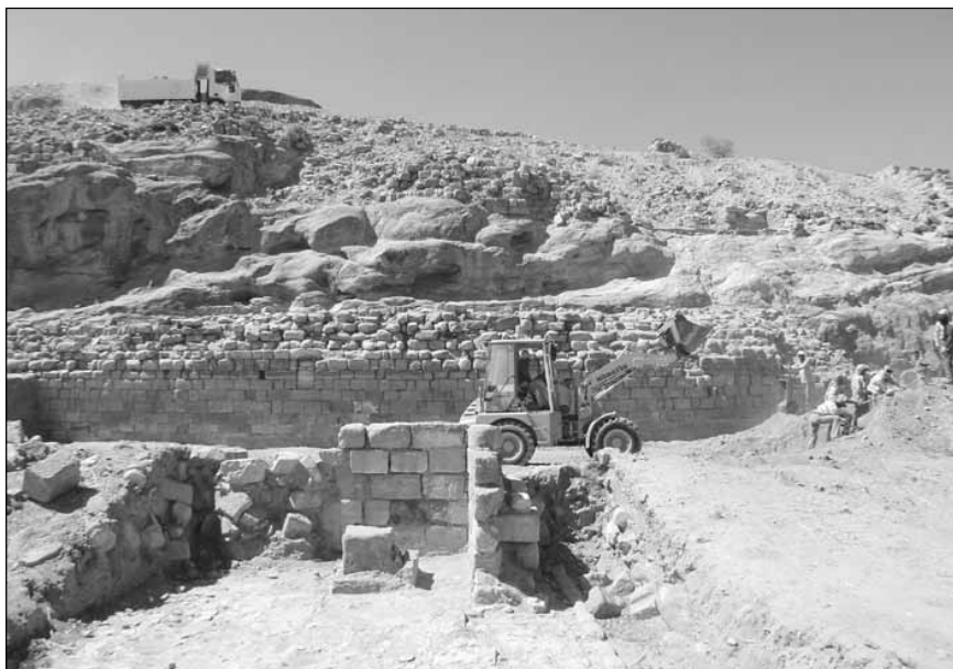
3. Removal of excavated overburden from the site with a backhoe and dump truck; island-pavilion in foreground.
